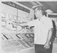
Antonio G. Geerman, Light Ends Panel Operator at the Refinery Operation Controlhouse here injects steam into the flare system to reduce smoke emission.
